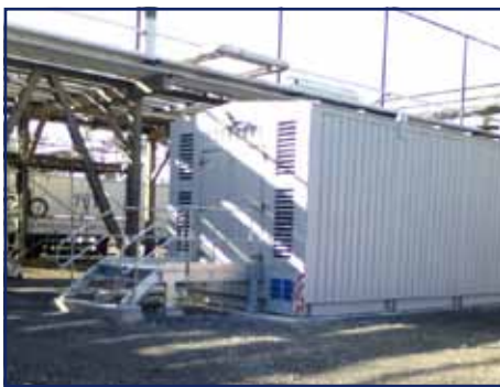
▲ Burner Management Project
